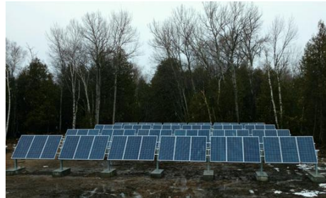
CBS Solar is currently installing our first Sell-All Project in Northern MI
