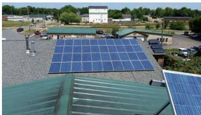
Pub racking by Patriot Solar
